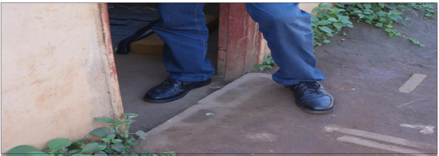
Figure 7: Example of poor substructure in low-income houses
