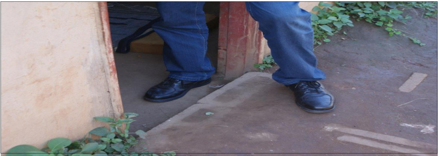
Figure 7: Example of poor substructure in low-income houses
