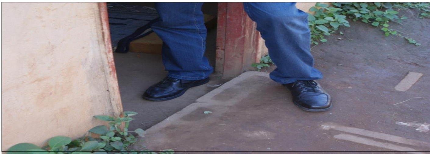
Figure 7: Example of poor substructure in low-income houses
